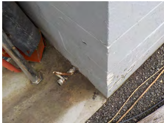
Containment drain valve.
