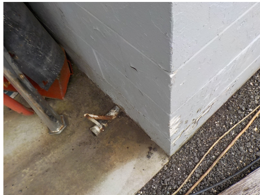
Containment drain valve.
