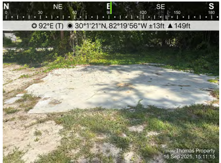
PHOTOGRAPH 8 View of the concrete foundation from the former residence on the east portion of the subject property.
