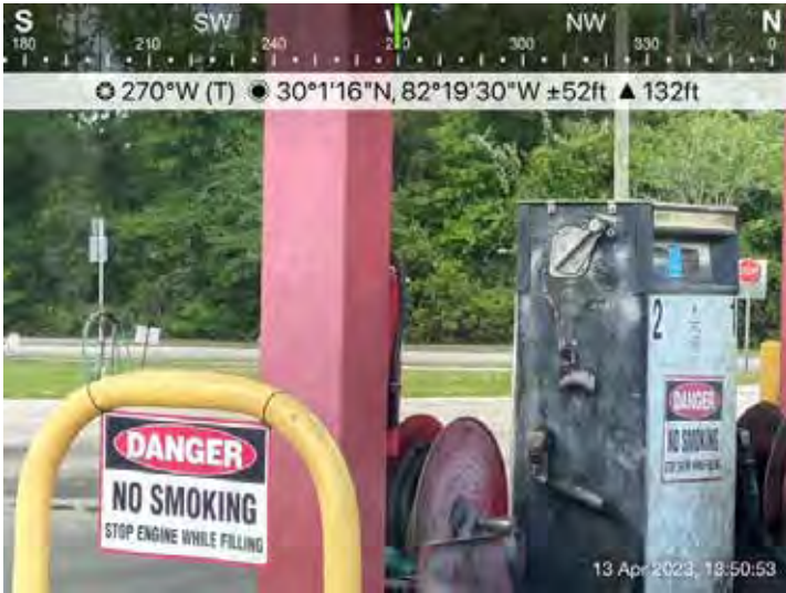
PHOTOGRAPH 9 Pritchett Trucking Fueling Station Pump Dispenser
