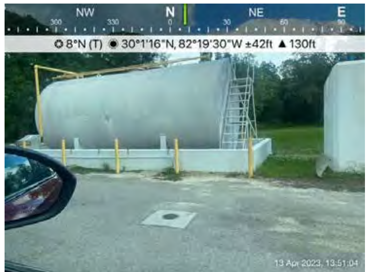
PHOTOGRAPH 12 Pritchett Trucking Fueling Station AST
